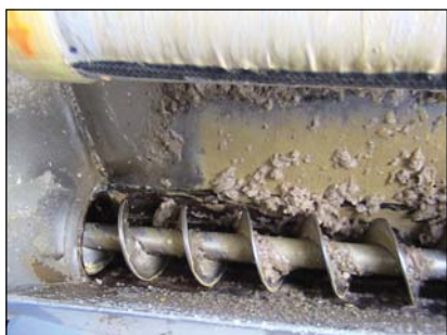
In the hopper, a screw press dewateres the solids to a cake with up to 40% solids.
